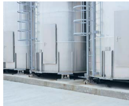
Tank & Hopper Weighing
